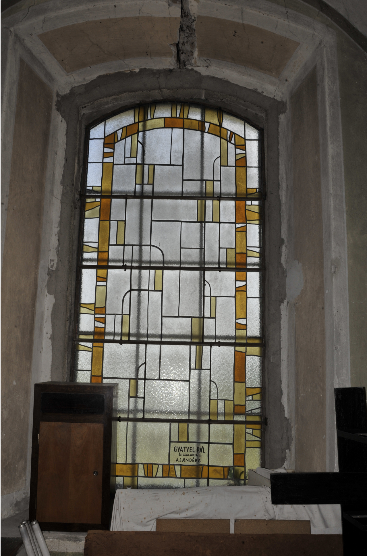
75/1 Templom ablak feleti repedés/ Crack above the church window
